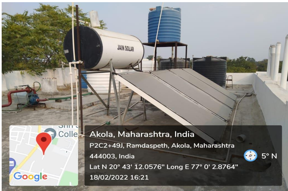
Solar Water Heater for Girls Hostel
